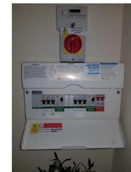
Example 1. Fuse board and isolation switch
