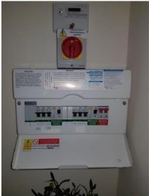
Example 1. Fuse board and isolation switch
